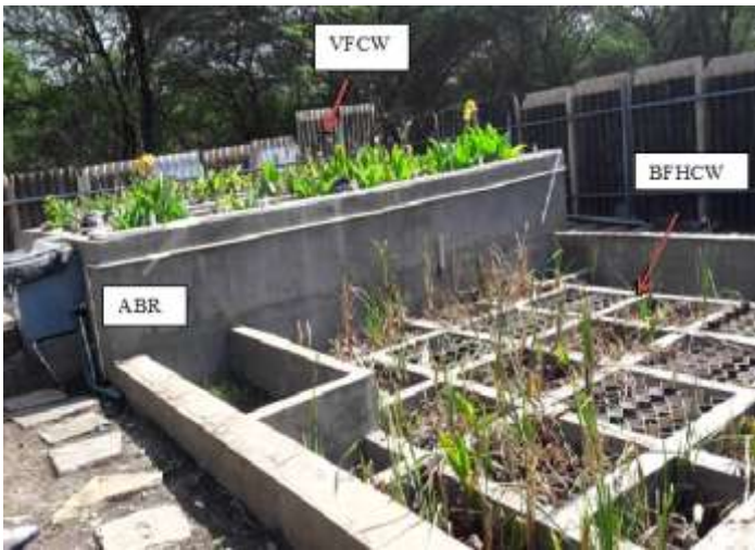
Figure 1: Photographic view of IDWTS at WCE, Sangli.
