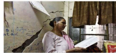
A woman checks cracks on the walls of a house due to the operation of Underground Metro Line, at Bahadur Puri, in New Delhi. (ANI/PTI)
