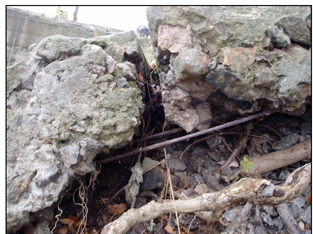
Fig. 3. Damaged area of the waterside protection.
